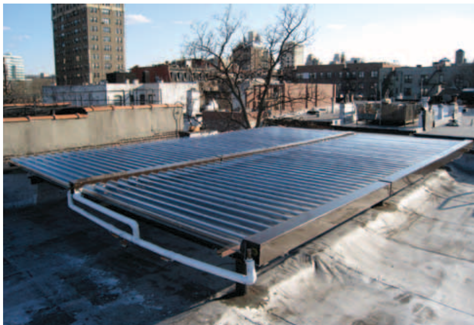
Solar Thermal System on roof of 176 Sterling Place. Notice load bearing wall on the right hand side of the system.
